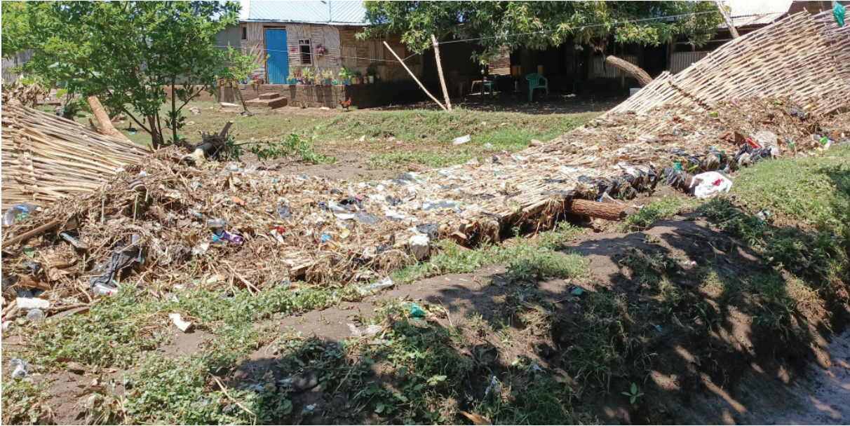
Fence damaged by flood
