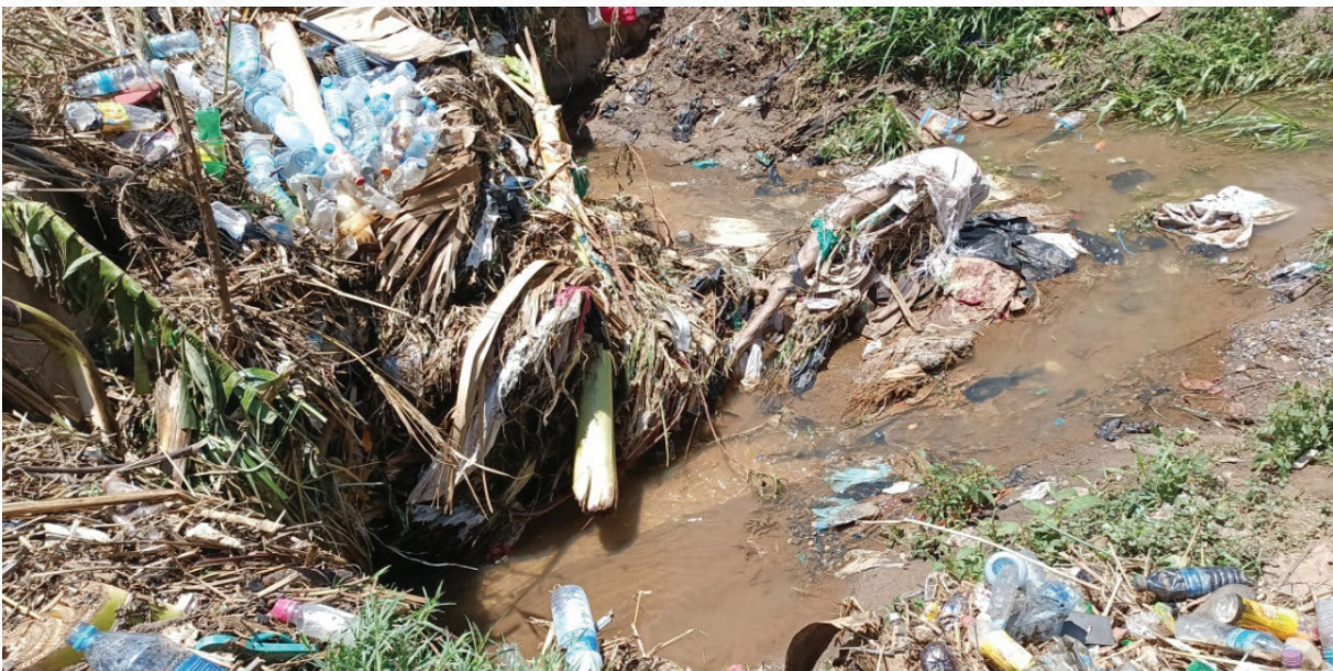
Culverts filled by wastes
